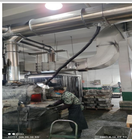
熔化炉渣罐口集气罩
